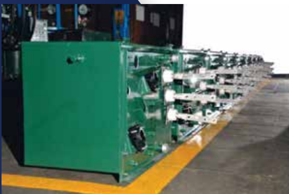
Accessory placement to the transformer
